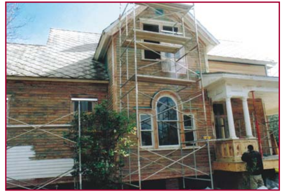
Terry Hayes' Restoration, exterior paint removal (using the #1 Paint Stripping System by Speed Heater)
