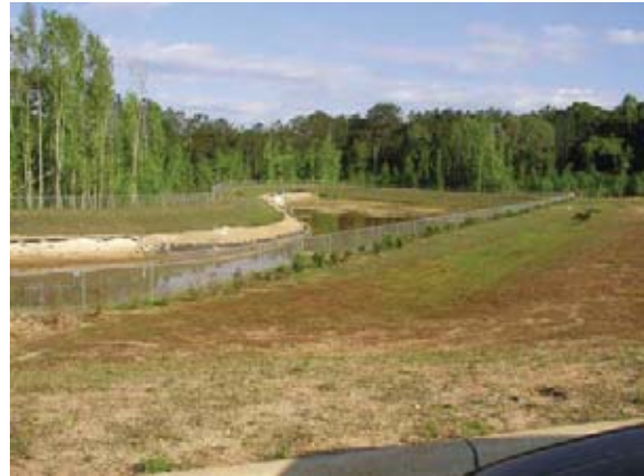
Pond with infiltration issues that does not drain properly
